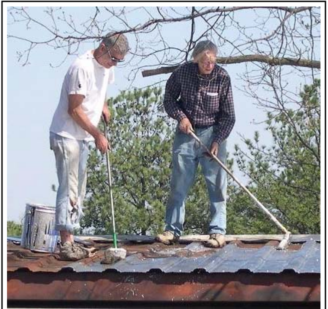
Phil Geary and Lew Southern painted the Pavilion roof. (They're 20+ feet above the ground!)
